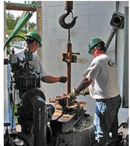
The well drillers install the tremie pipe to plug the geologic zone that contributed water heavy in radionuclides. Photos courtesy Boone County PWS #9
